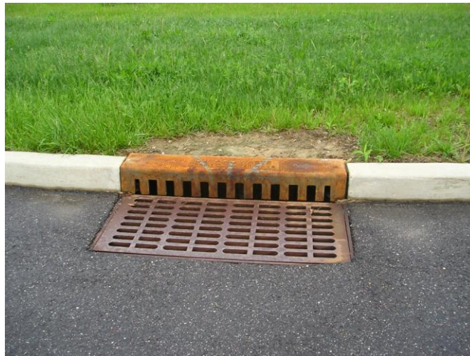
Storm Inlet in Conformance with Stormwater Ordinance
